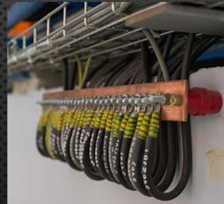
Phone Tower BUSS
